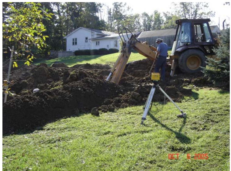
Installation of a new household sewage treatment system that received $4,000 cost share from the OEPA S.319 grant.
